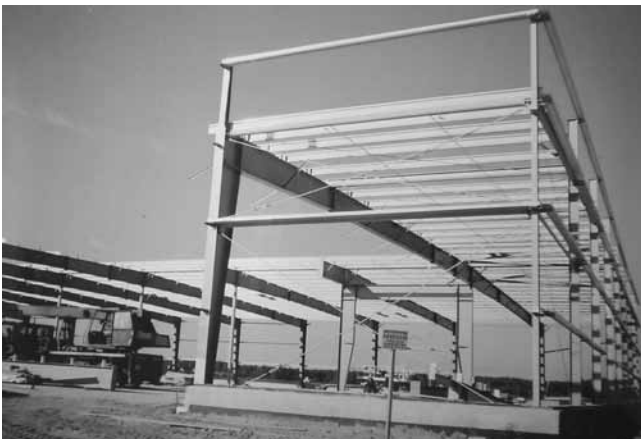
Rys. 7. Niezmontowane dwa przęsła hali, w których spoiny badano metodą UT Fig. 7. Two not-assembled severy bays of hall in which the welds using UT method were tested
